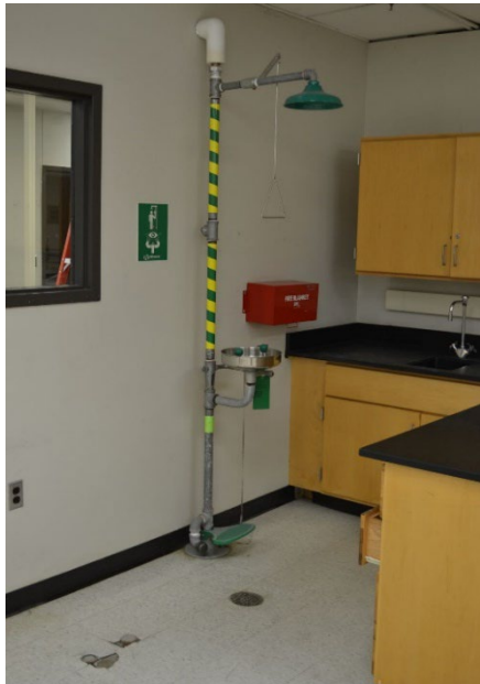
Emergency wash station
