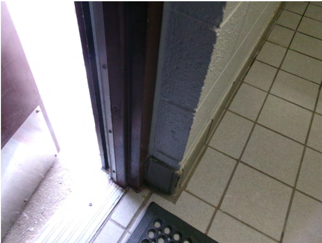
9d4 Women's room rusted door frame
