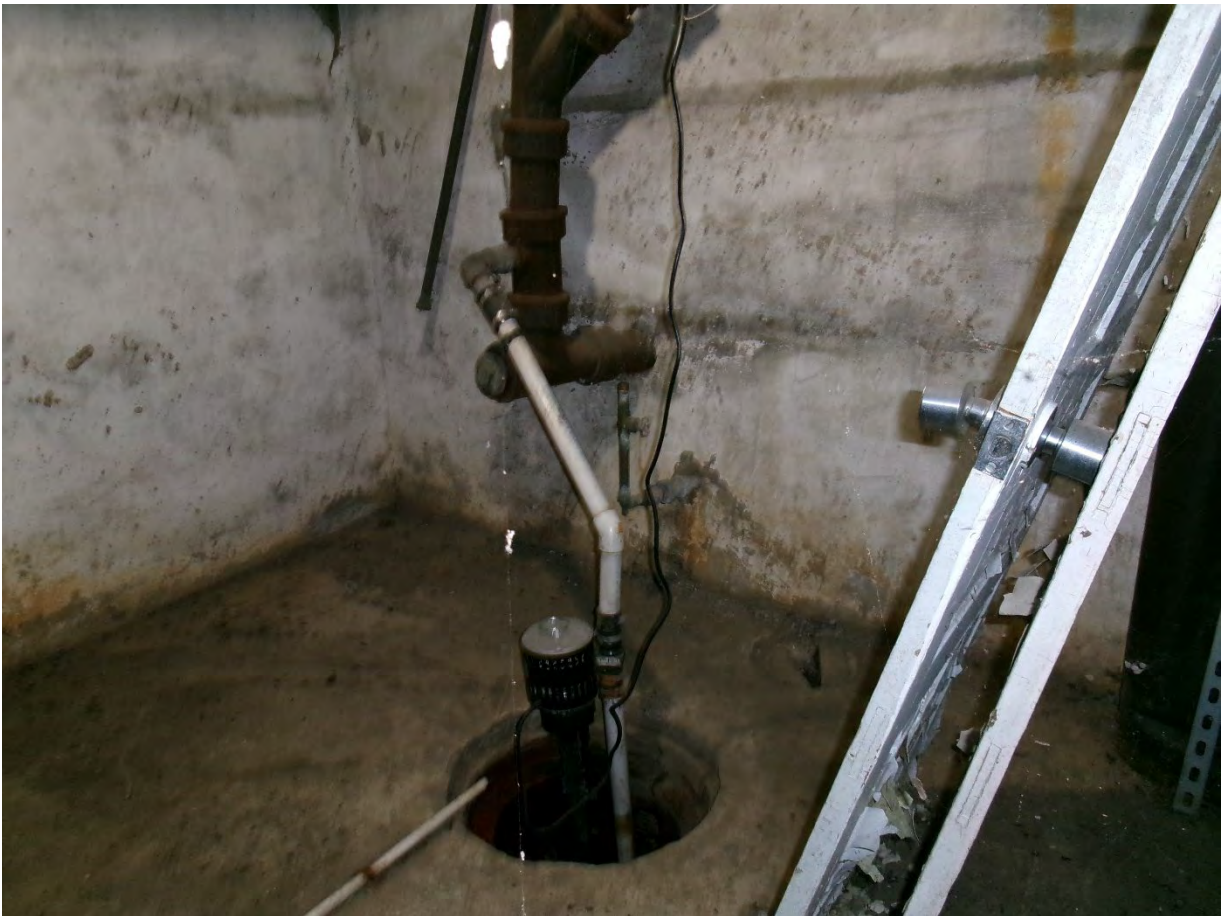
7f16 New sump pump
