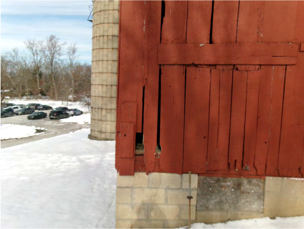
8c3 Exterior wall siding gaps
